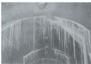
乌江渡水电站大坝灌浆廊道中发育的鹅管 Secondary sediment developing in Wajiangdu Hydropower Station dam's grouting gallery
